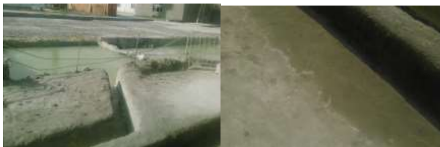
Pic. 1. Sewage treatment plant of slate production.
